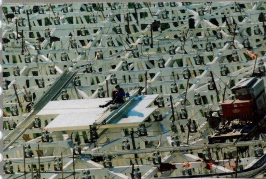
* GBT 09/23/98 (13) Looking E. GBT Site. Tim Weadon testing the panel adjusting tool.
