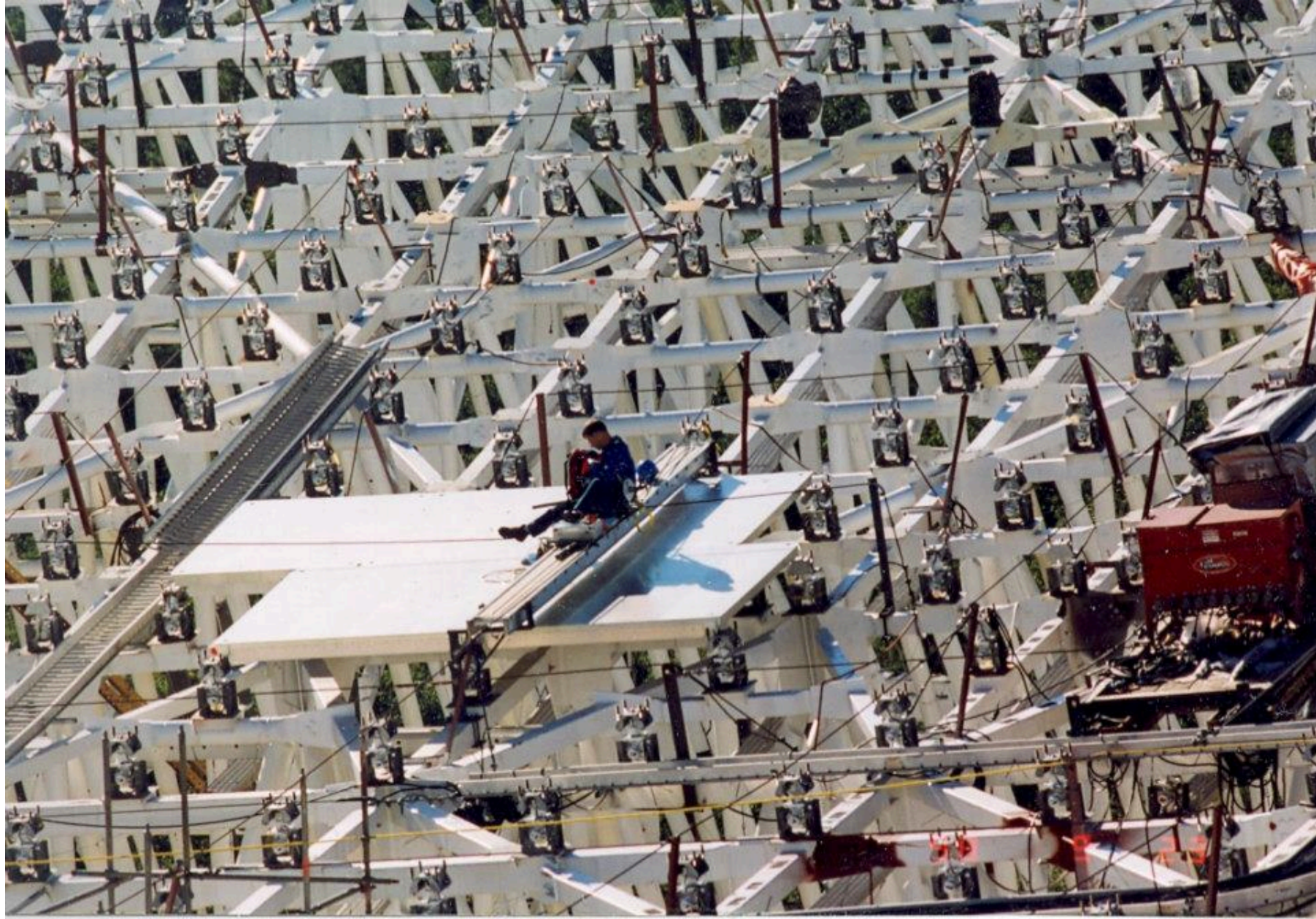
* GBT 09/23/98 (13) Looking E. GBT Site. Tim Weadon testing the panel adjusting tool.
